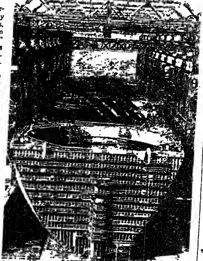
A tanker for liquefied natural gas during construction in the General Dynamics yard in Quincy, Mass.
